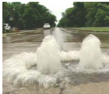
Sewage overflowing a manhole due to an overloaded sewer.
